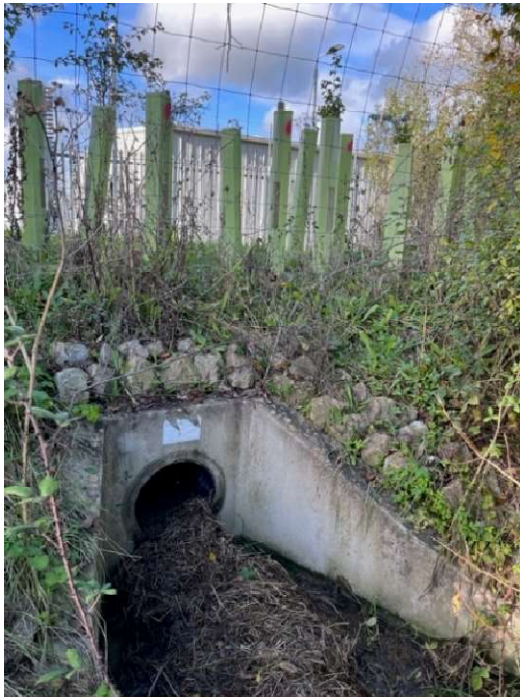
Rampion 1 Substation, dry ditch
